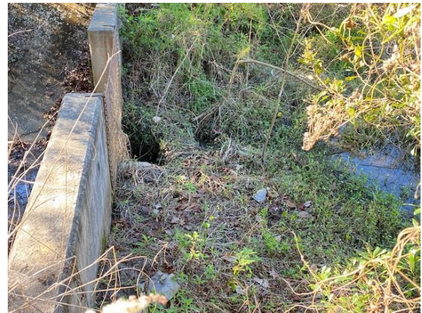
Channel in front of concrete weir needs to be desilted to function properly.
