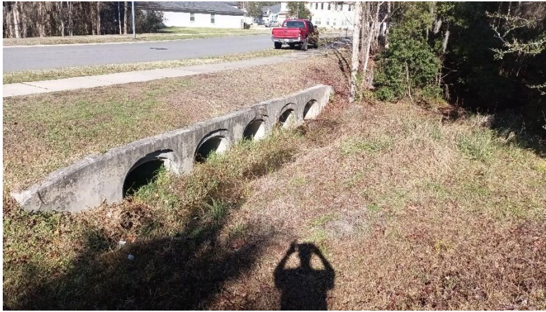
Needs clearing and silt removal. Same as 2023 Report.
