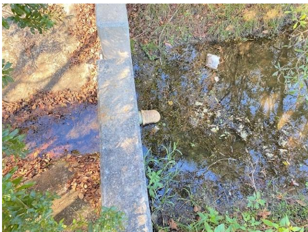
Channel in front of concrete weir needs to be desilted to function properly.
